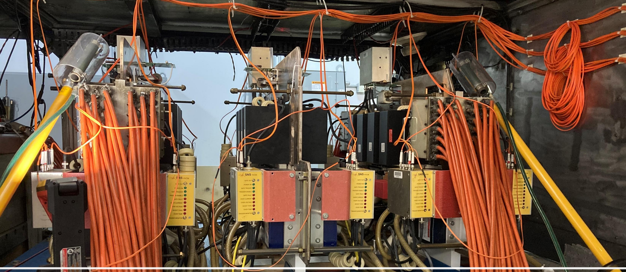
SNS HVCM – Safety Enclosure
