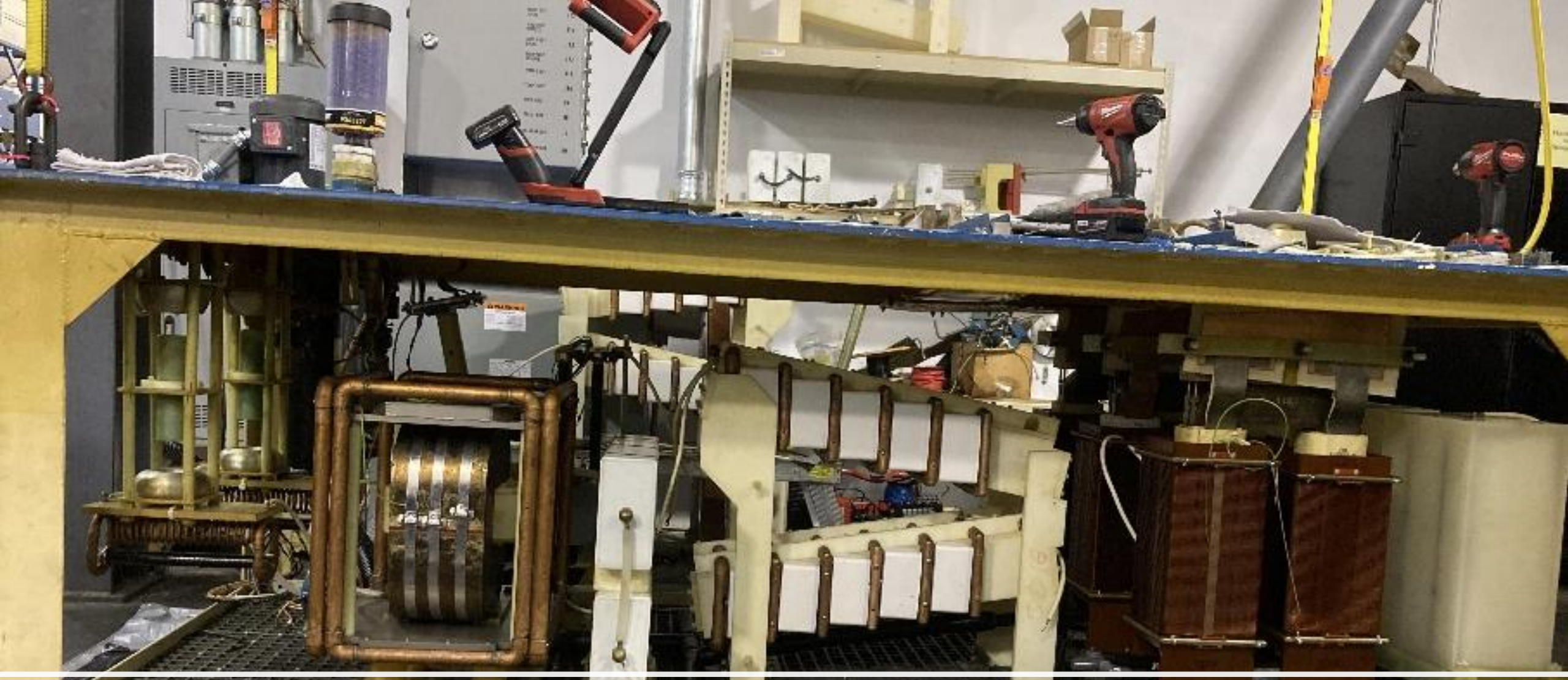
SNS HVCM – High Voltage Oil Tank
